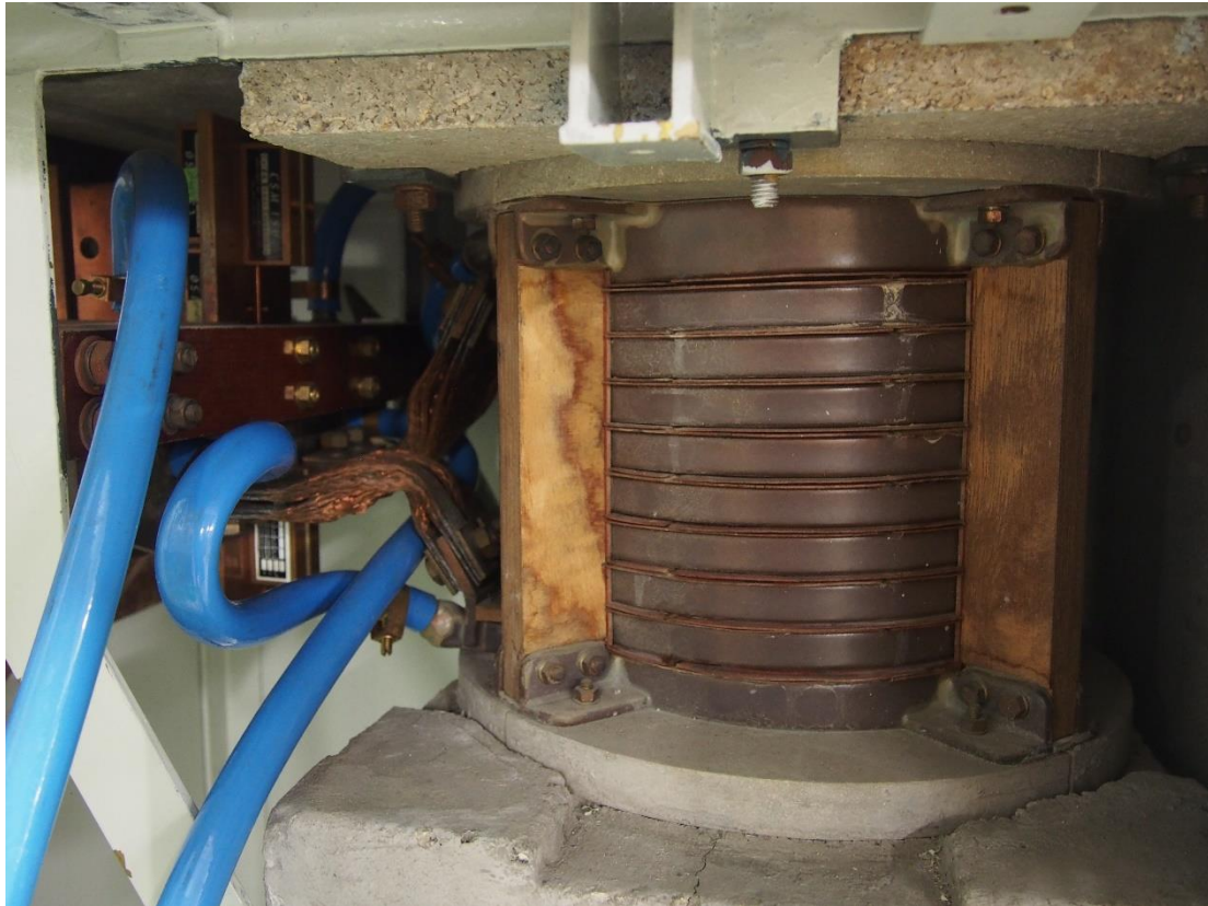
Figure 5.1: detailed view of the induction crucible furnace. Copper inductor and capacitors bank
